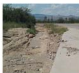
Damage at Wilmont and Sahuarita Rd. due to flood waters
